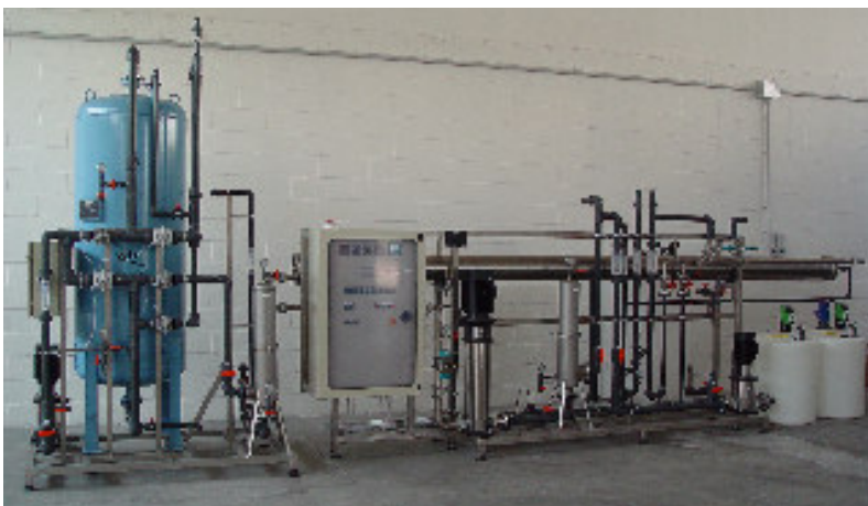
Example of a reverse osmosis system complete with pre-treatment: bi-layer filtration, dosing of chemical agents.
